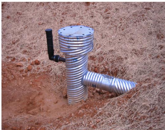
Figure 7.31-6 Dewatering device on Riser with Trash Rack
